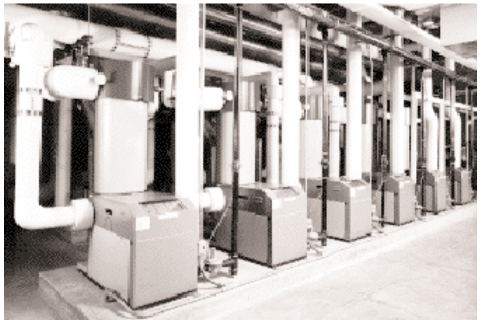
Figure 2. Typical Multi-Unit Water Heater and Hydronic Boiler Installation (photo courtesy of Aerco International, Inc.)
